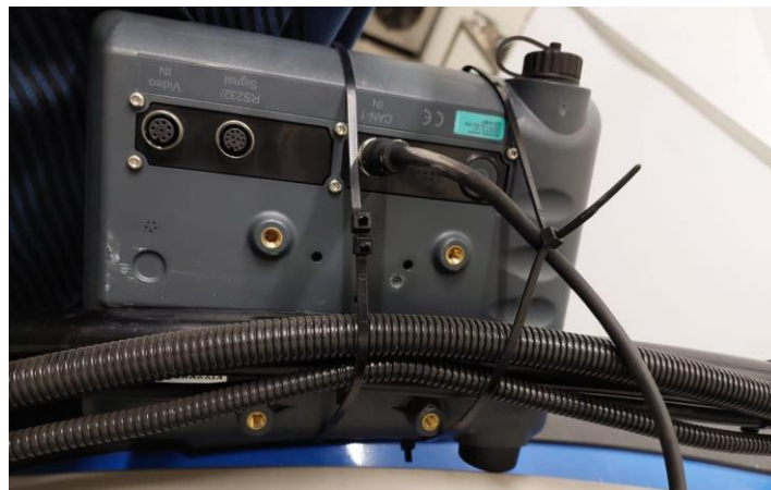
Figure 13: VT terminal is still mounted with tie wraps
